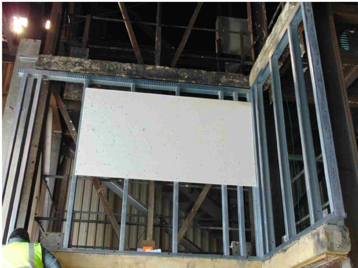
Figure 4. Lightweight steel framework partition between floor slabs with single sheathing board fitted.
