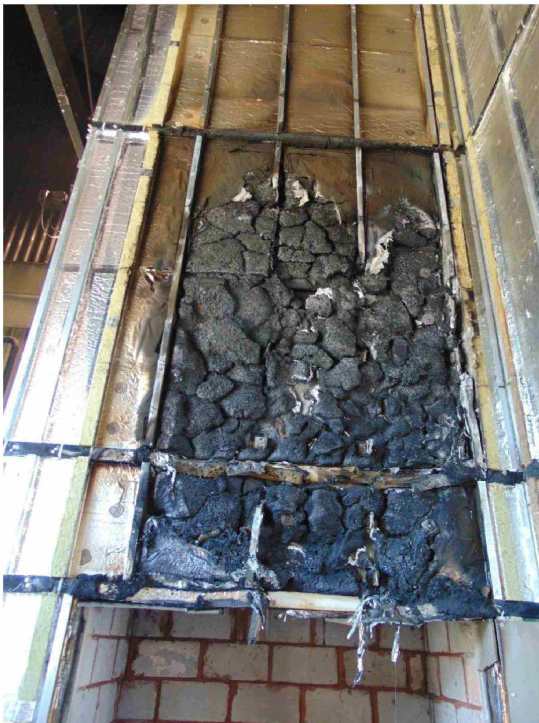
Figure 29. Post-test close up of main wall insulation, rail substructure and cavity barriers above the combustion chamber opening.
