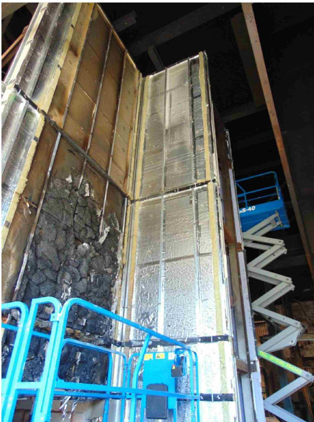
Figure 288. Post-test wing wall view of insulation, rail substructure and cavity barriers from the top of the combustion chamber to the top of the cladding system.
