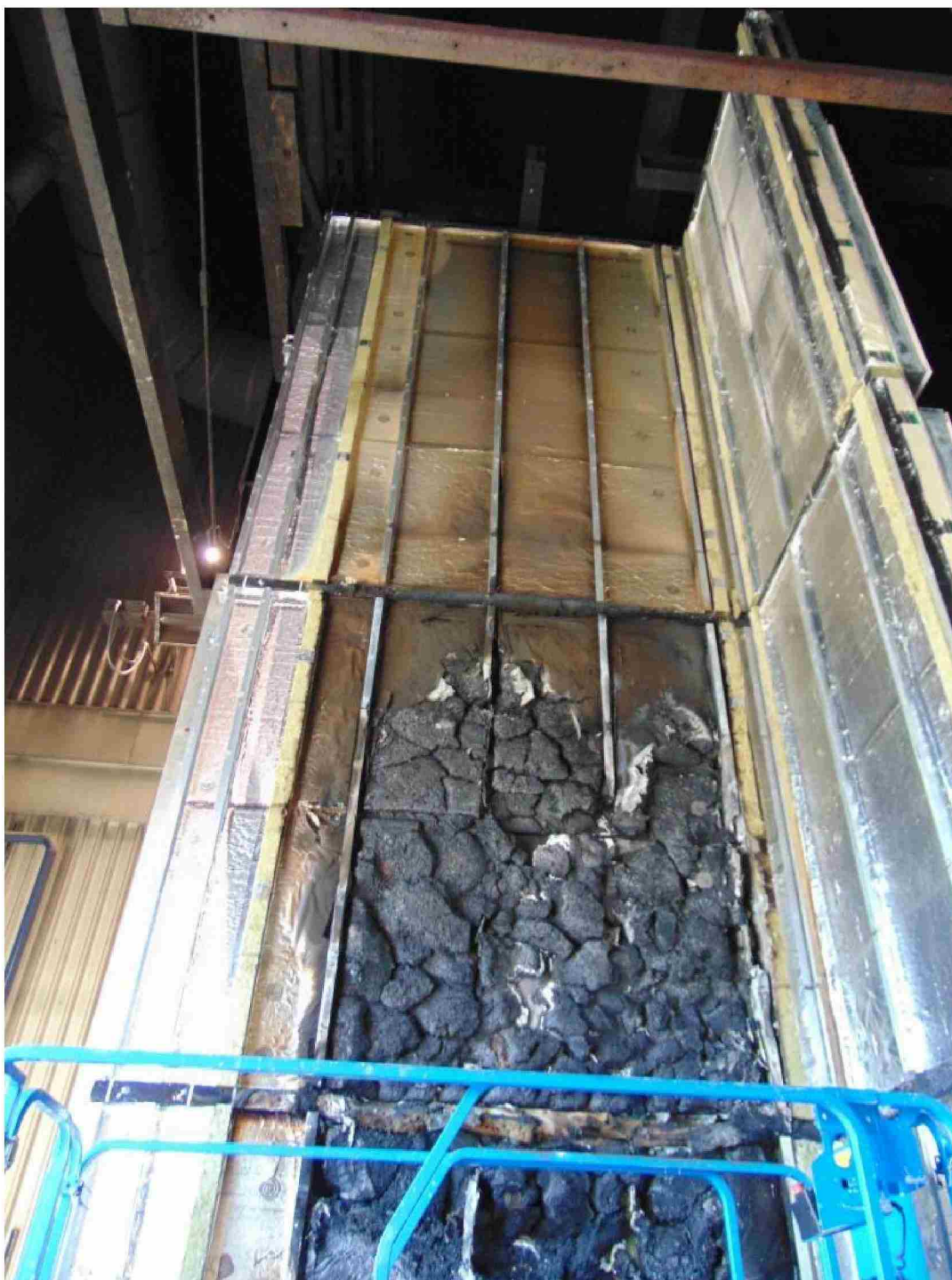
Figure 277. Post-test main wall view of insulation, rail substructure and cavity barriers from the top of the combustion chamber to the top of the cladding system.
