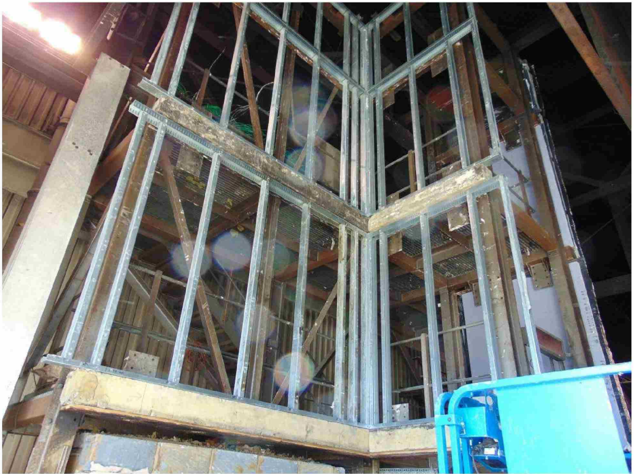
Figure 32. Post-test view of lightweight steel framing system from the top of the combustion chamber to the top of the cladding system.
